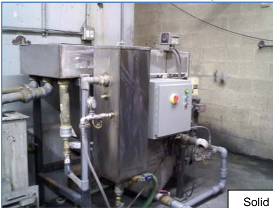
Lamella Flow Clarifier on Wash System
